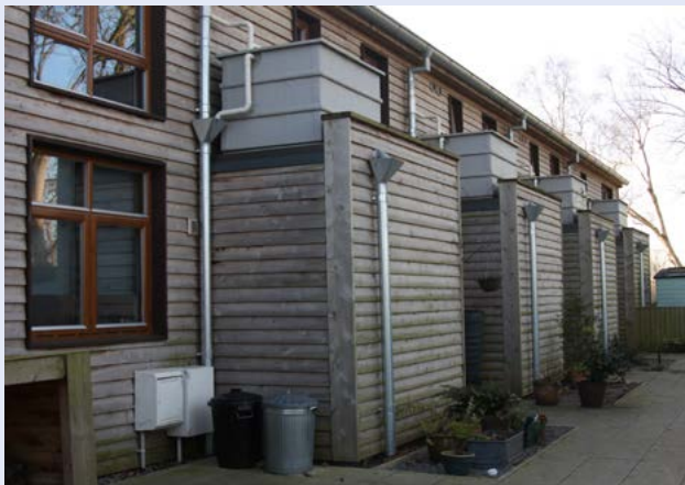
FIGURE 25: HOME RAINWATER CAPTURE SYSTEMS
